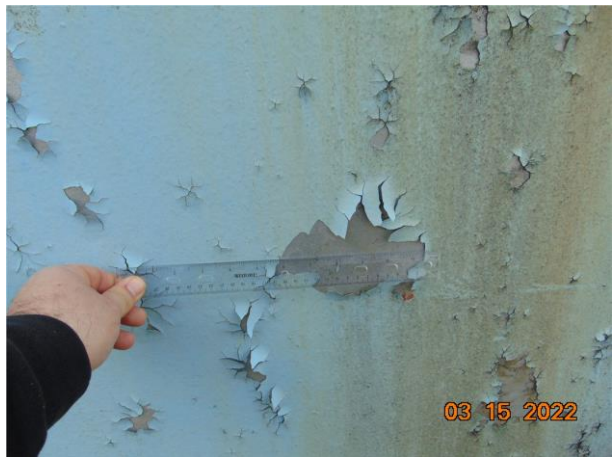
8) Delaminated shell coating
