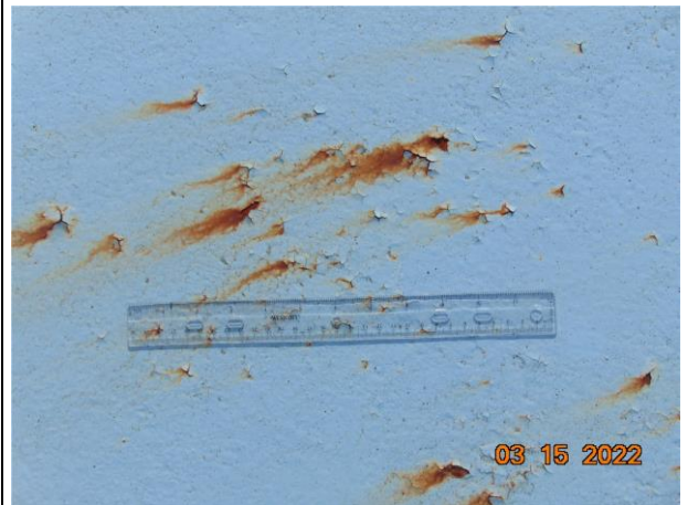
11) Corrosion the roof plates
