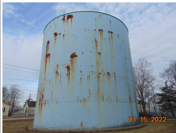
2) Corrosion on the shell
