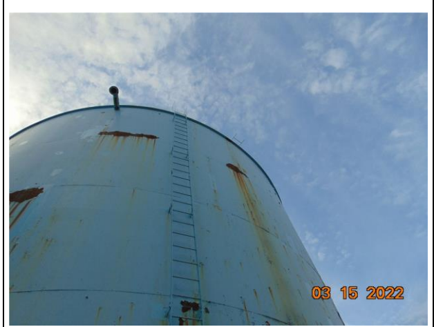
4) Ladder and overflow
