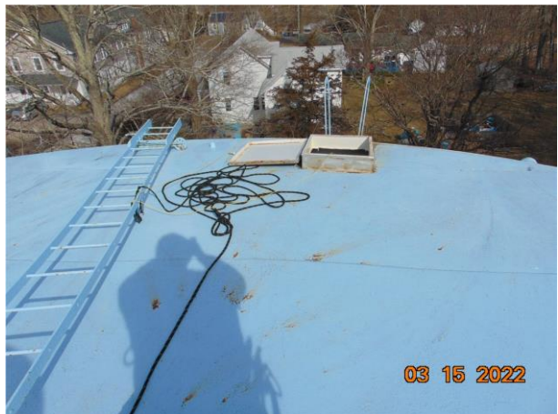
9) Roof hatch, roof ladder, roof plates
