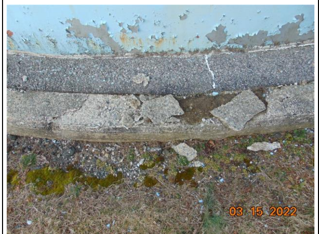
6) Cracking on the foundation
