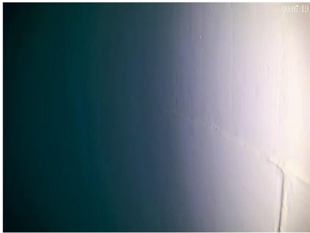
26) 07:27 Typical shell condition
