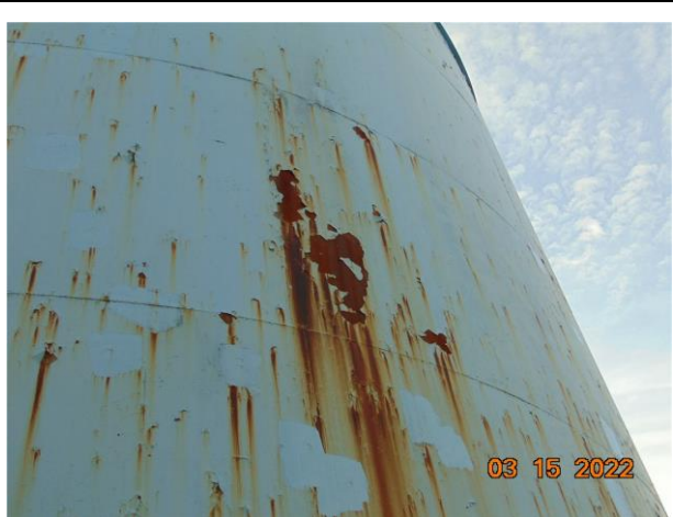
7) Coating delamination with corrosion
