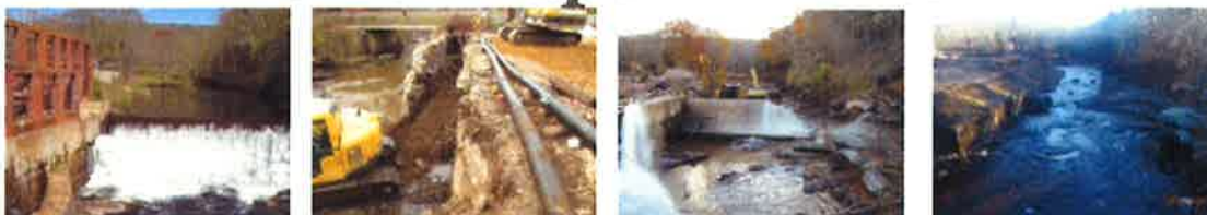
Before and after photos show the removal of the Norton Mill dam on the Jeremy River.
